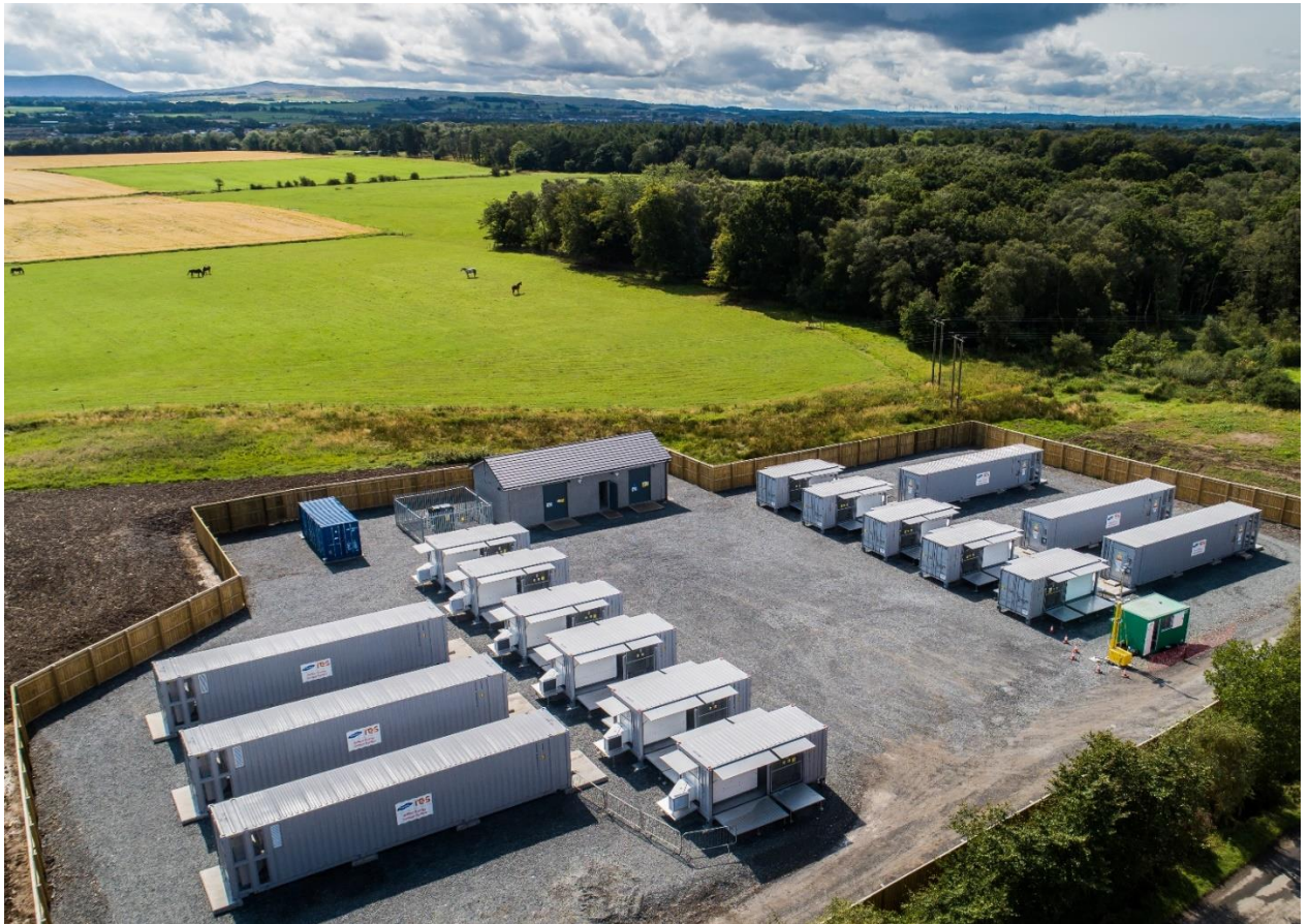
Diagram 8: Aerial of Battery Energy Storage System (BESS) at Broxburn Wind Farm by Keith Arkins
